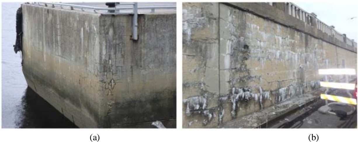
Figure 2: (a) Moderate AAR cracking in cope wall and (b) More severe AAR cracking gel discharge in retaining wall (Alexander, 2019)
