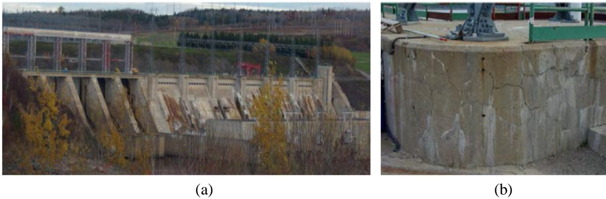
Figure 11: (a) Mactaquac Dam in Canada exhibiting map cracking in 2008; (b) Cracking on dam elements (Thomas, Folliard, et al., 2017)
