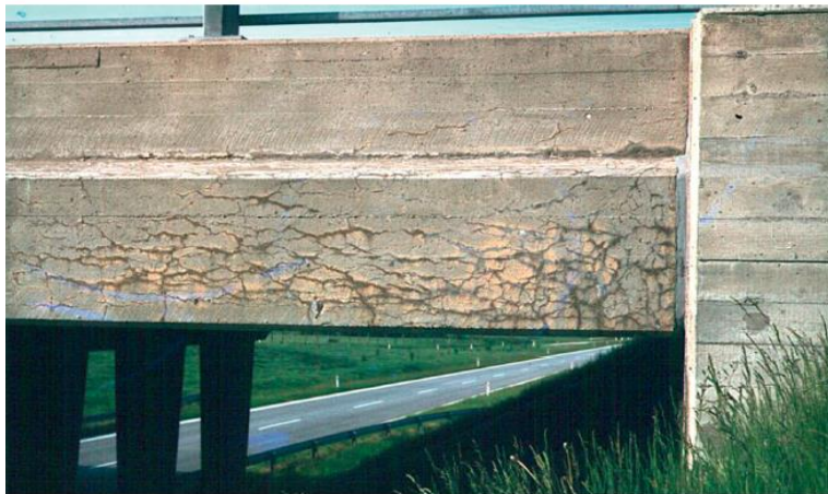
Figure 19: Cracking due to ASR on a bridge in Ølstykke in Denmark (Lindgard et al., 2017)
