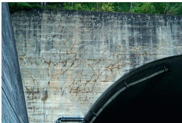
Figure 21: Tunnel showing dense cracking pattern in Switzerland (Fernandes et al., 2017)
