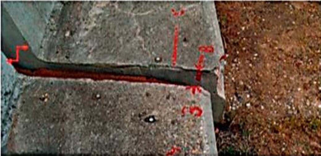
Figure 18: Large concrete block in a dam in Australia displaced (Shayan & Freitag, 2017)
