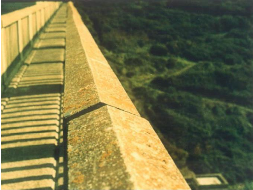
Figure 4: Concrete parapet of the Val de la Mare Dam in the United Kingdom with a displacement of up to 13mm (Sims, 2017)
