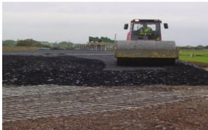
Figure 2.53 – Steel reinforcement cage under embankment LTP for LGV project Paris, Bordeaux (Coghlan, Plomteux & Racinais, 2016)
