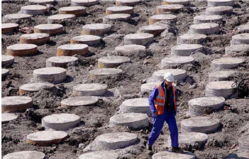
Figure 2.3– Rigid Inclusions (Vibro Concrete Columns) in a rectangular grid pattern (Balfour Beatty, 2016)
