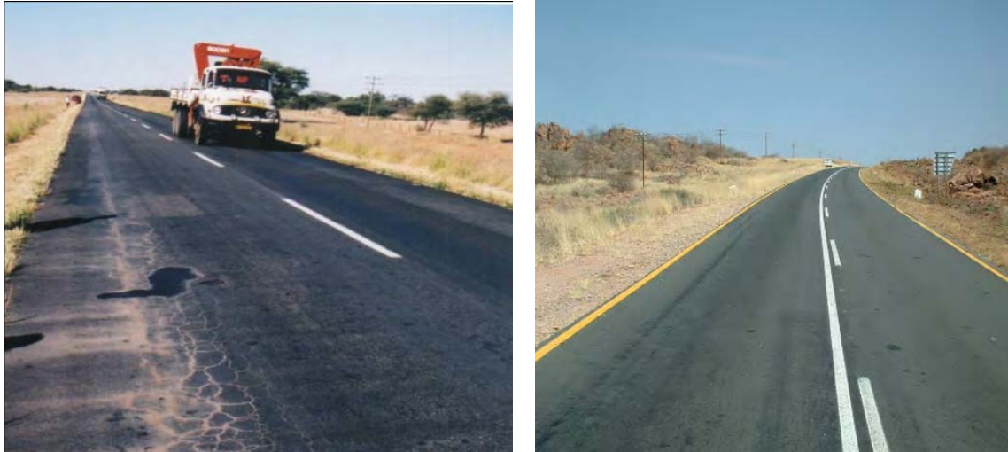
Figure 17 : A) Road with pavement failure B) Road with gravel shoulders
