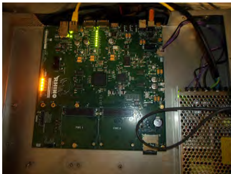
Figure 6.25: Loading configuring the RHINO with the gpmc_test.bof gateway design illustration from the command line and the RHINO board
