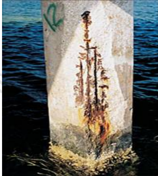
Figure 1.1: The effects of steel reinforcement corrosion in a bridge pier
