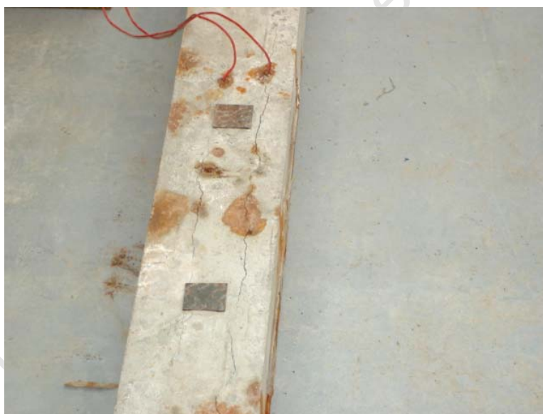
Figure 5.10: Longitudinal cracks due to corrosion of the steel reinforcement
