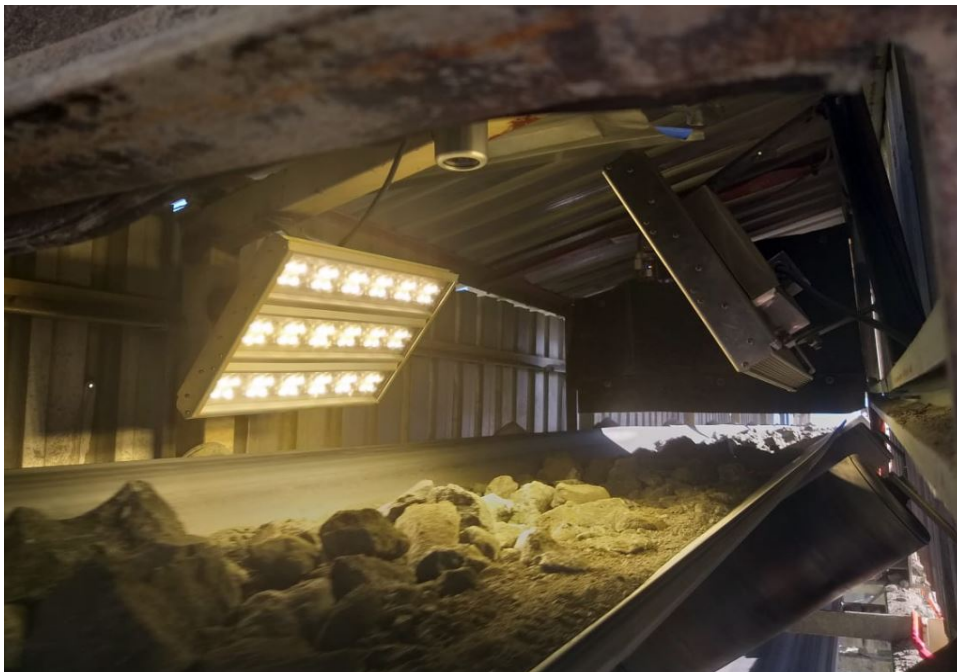
Figure 4.3: Camera and floodlight installation at Kao Diamond Mine, above the primary feed conveyor.
