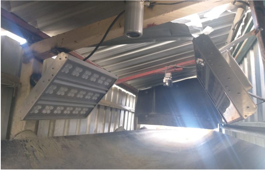
Figure 4.1: Camera and floodlight installation at Kao Diamond Mine, above the primary feed conveyor.
