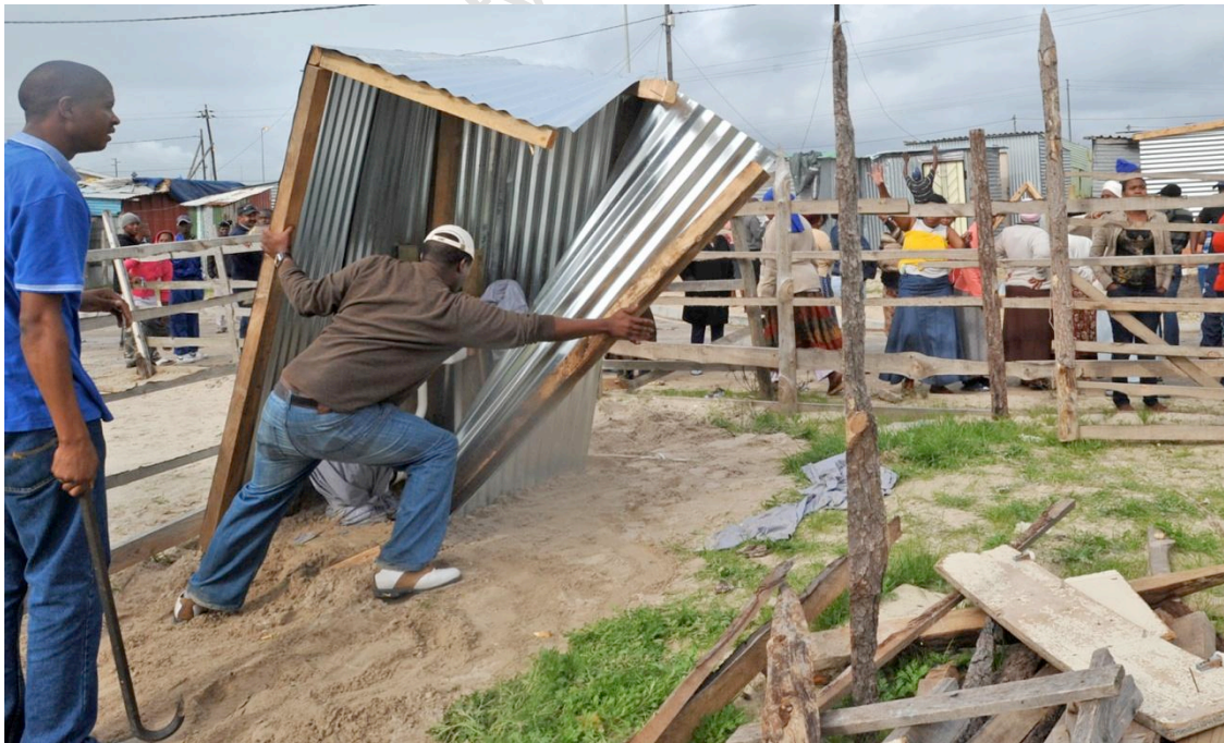
Residents Breaking Down the Corrugated Enclosures Provided by the City Council (Courtesy Independent Newspapers)
