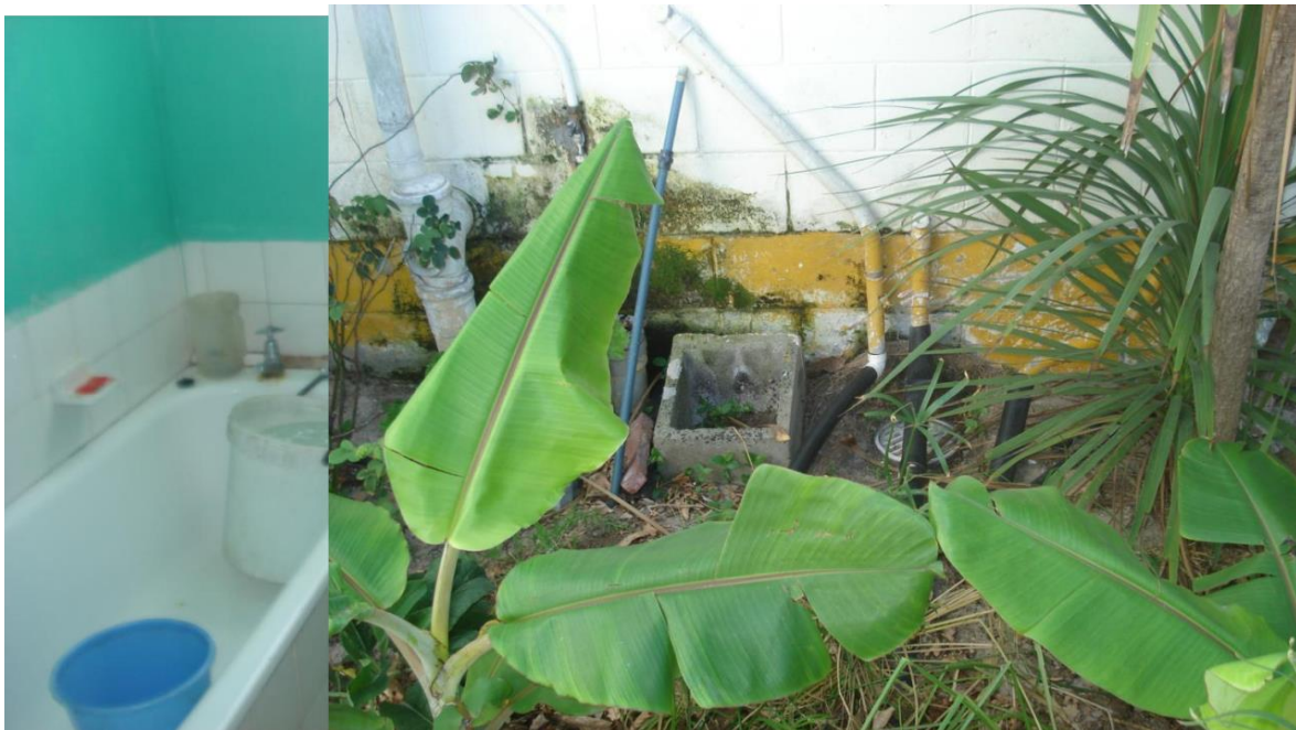
Figure 2: Grey water recycling system with papyrus plants for water filtration with pre-existing banana trees in the foreground
