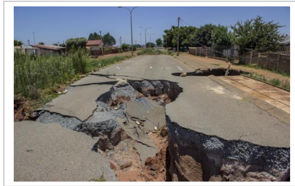
Figure 2.2: Ground subsidence in Gauteng resulting in destruction of road infrastructure and sanitation system (Image by Delwyn Verasamy).
