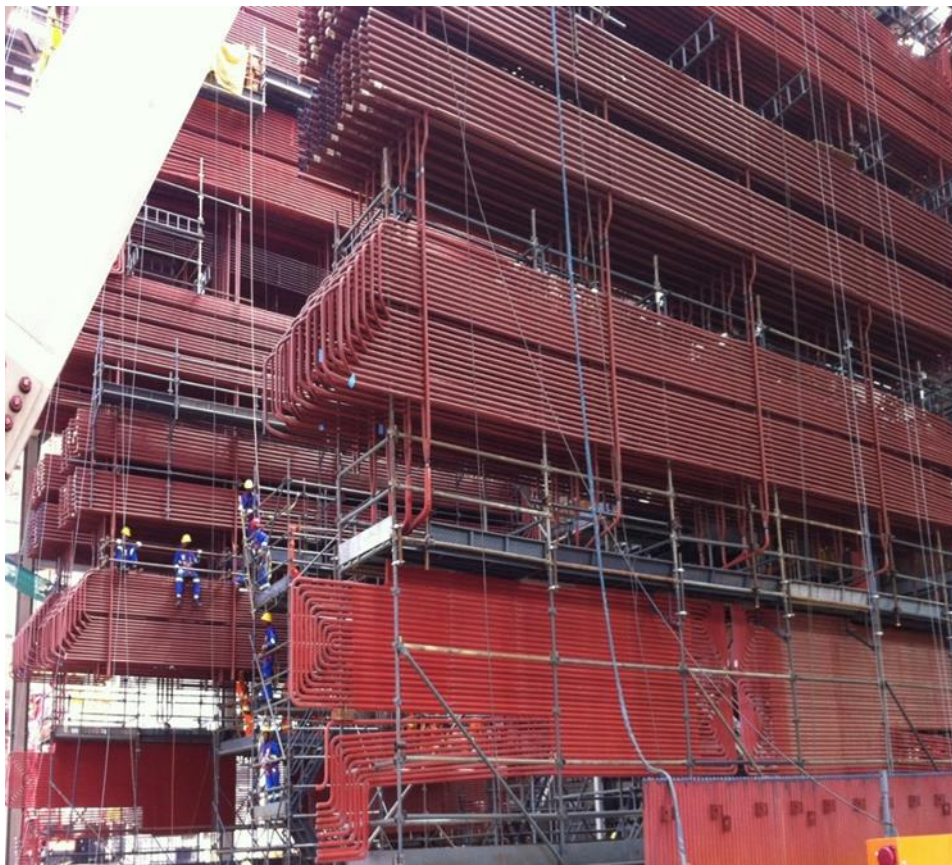
Figure 2-4. Tube banks for the superheaters and reheater in a once through 800 MWe boiler system.
