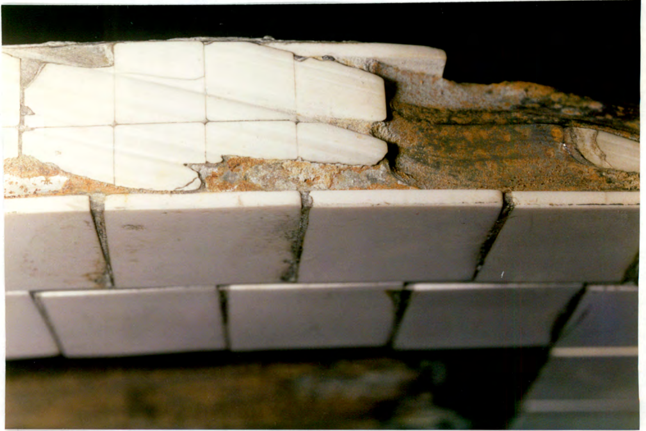
Figure 3.22 Degradation of underlying metal once protection by ceramic tiles is lost.
