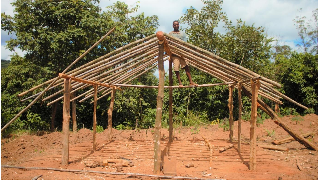
Figure 124. This photograph that I took in 2017 in Nvava shows Mwene Mpida's new house being constructed with the help of one of his nephews using local forest materials.
