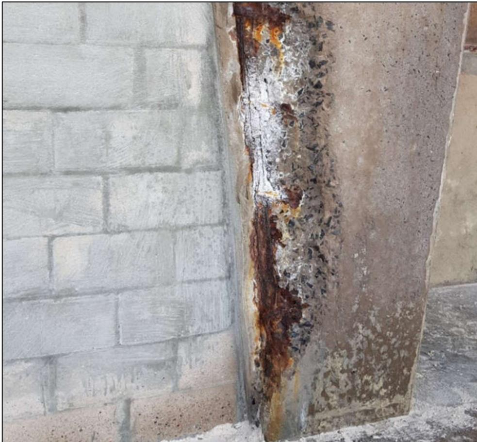
Figure 2-4: Chloride-induced corrosion of a reinforced concrete member in a coastal environment
