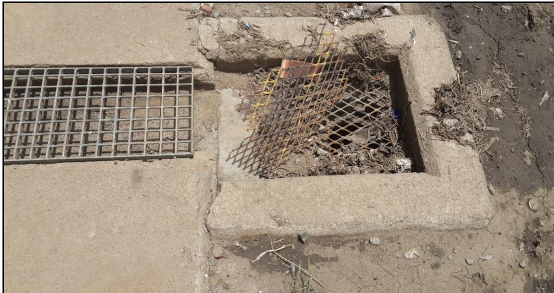
Figure 42: Missing Drainage Catch Pit Cover Grid
