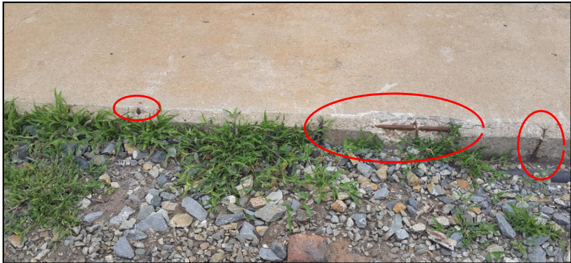
Figure 39: Spalling on the edge of floor slab
