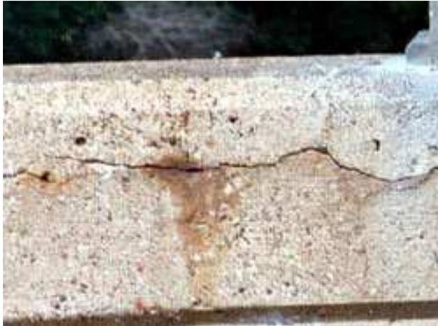
Figure 2.2: Corrosion crack longitudinal to reinforcement direction ( www.cement.org/tech/faq_cracking.asp , 2009)
