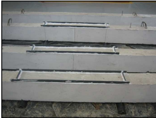
Figure 3.6: PVC corrosion ponds on concrete beams
