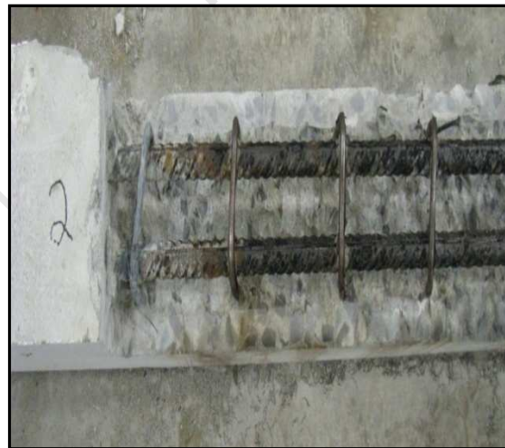
Figure 3.8: Reinforcing steel after cleaning corrosion products
