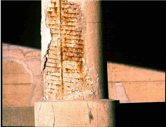
Figure 2.1: Corrosion of steel reinforcement ( http://irc.nrc-cnrc.gc.ca/ircpubs , 2004)
