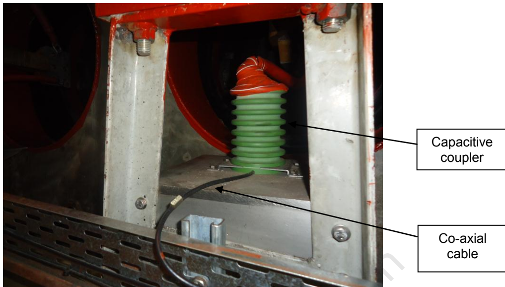
Figure 3.7: Capacitive coupler with co-axial connection for transfer of high frequency of PD signal
