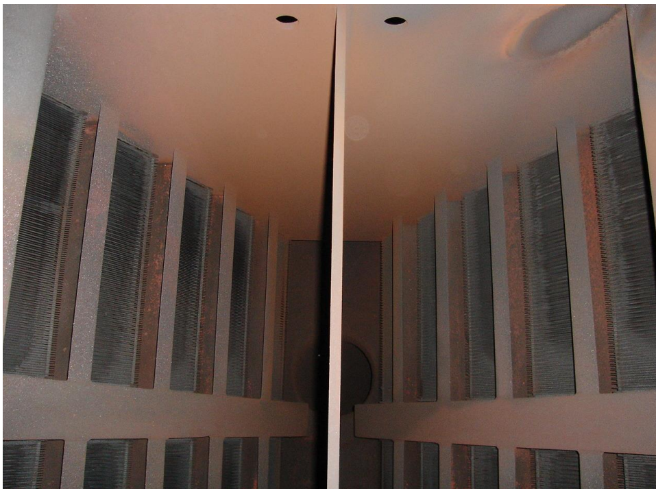
Figure 20: Moisture separator blocks in vessel, viewed from the manway at the top of the vessel looking down [undisclosed source]
