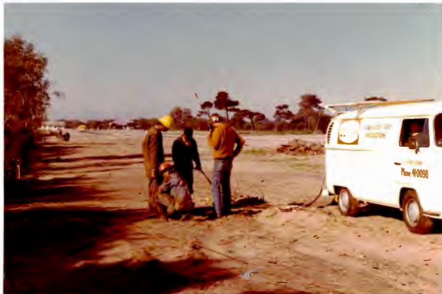
FIGURE 11: THE TELEVISION CAMERA BEING USED TO INSPECT 150mm SEWER PRIOR TO ACCEPTANCE FROM CONTRACTOR.
