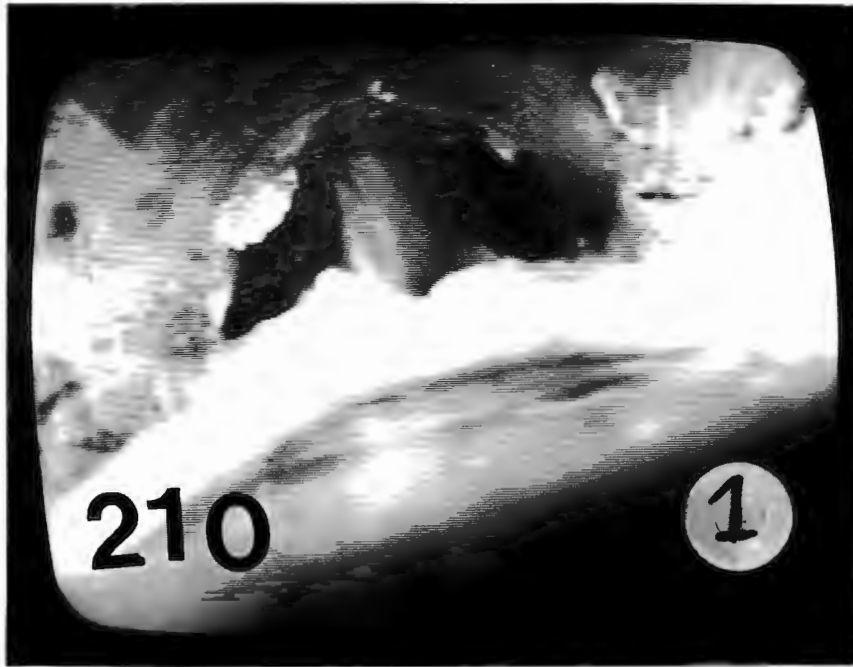
FIGURE 6: INDUSTRIAL DISCHARGE WITH DETERGENT - 300mm SEWER, AUCKLAND STREET, PAARDEN EILAND.
