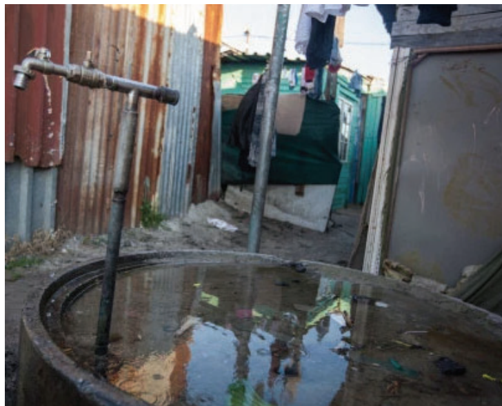
Figure 7: A communal water tap in Khayelitsha. Photo by Shachaf Polakow
