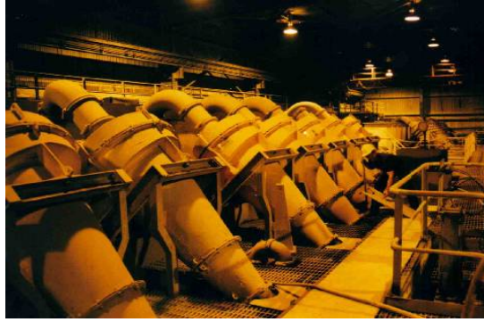
Figure 2-19: Picture showing inclined cyclones in a processing plant.
