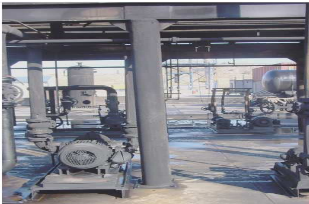
Figure 2.2: Permanently deformed column caused by different temperature between the west and east face [17].
