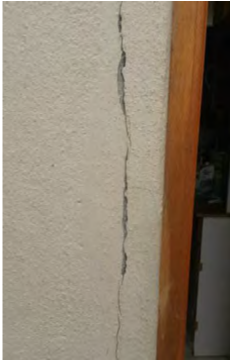
Figure 4.9: Cracked Walls (Source: author's photographs)
