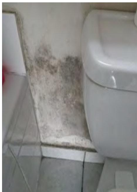
Figure 4.8: Damp Walls (Source: author's photographs)
