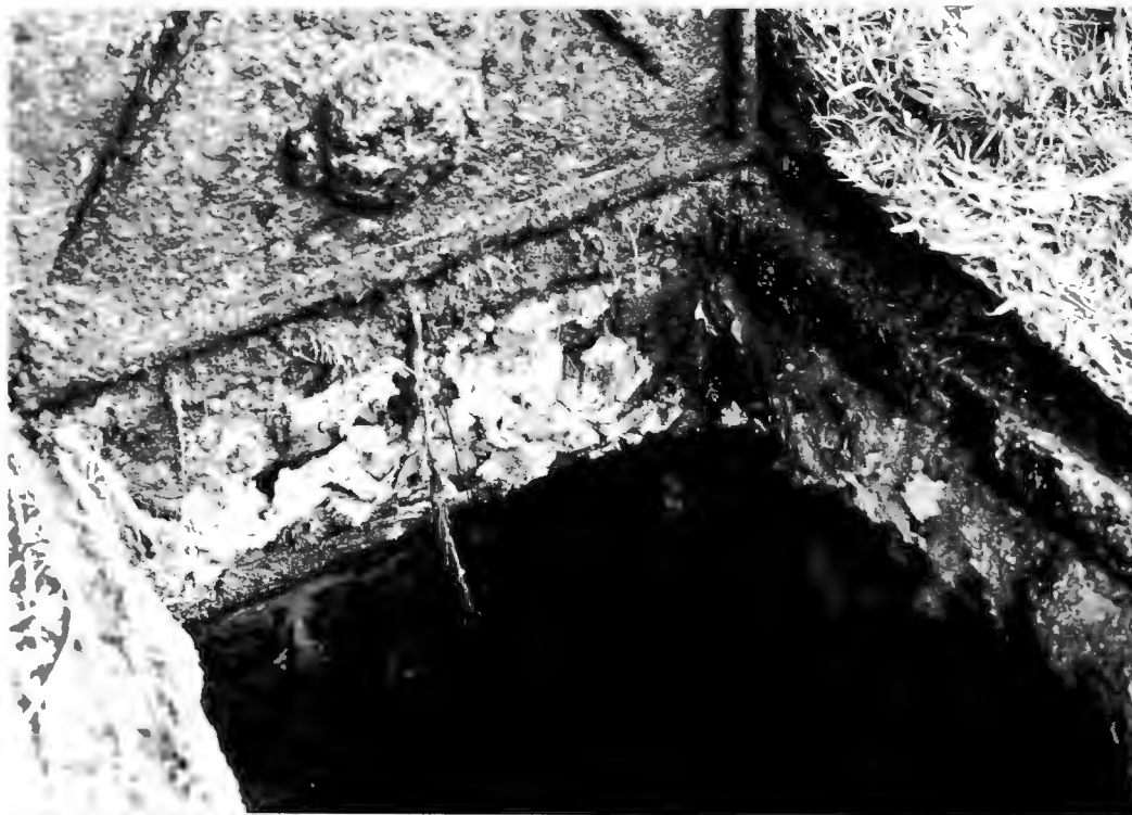
PLATE 1.1: Severe disintegration of the concrete roof slab of a septic tank and severe deterioration of the cast iron cover frame
