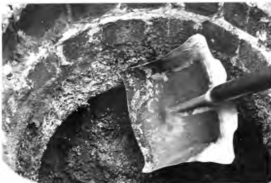
PLATE 1.2: Corrosion of the concrete roof slab yielding soft mushy material of negligible strength. (See vicinity of top left hand corner of the spade.)
