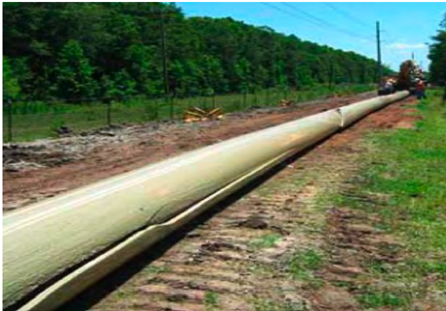
Figure 3-18: Rapid crack propagation in PVC pipe (Source: Long (2012))
