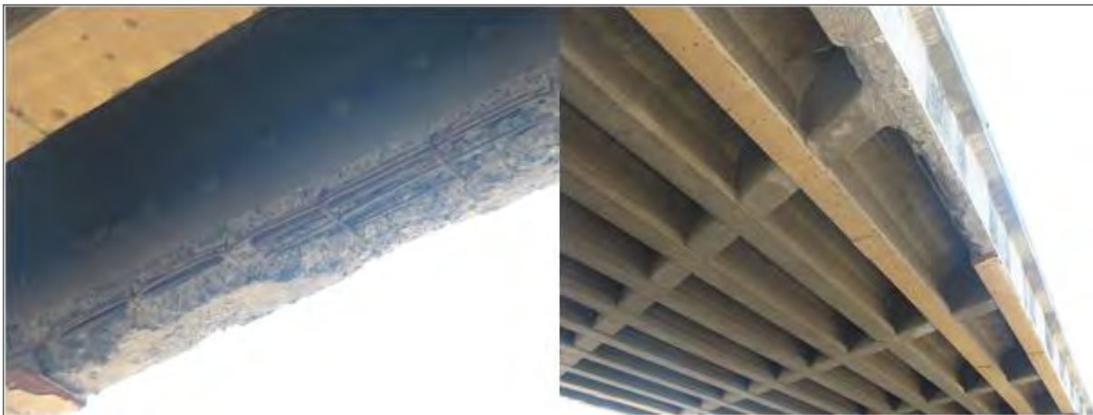
Figure 19: Bridge beam damaged due to transverse vehicular impact (SMEC, 2007)
