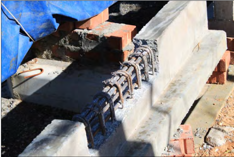
Figure 44: Exposure of bottom steel reinforcement
