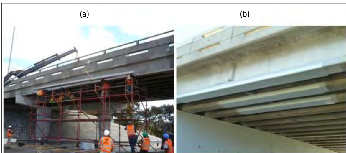
Figure 23: Damaged bridge beams strengthened using externally bonded steel plates a) scaffolding required for placement b) after completion (SMEC, 2007)
