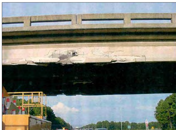
Figure 20: Severely impact damaged bridge beam (Chhabra, 2014)
