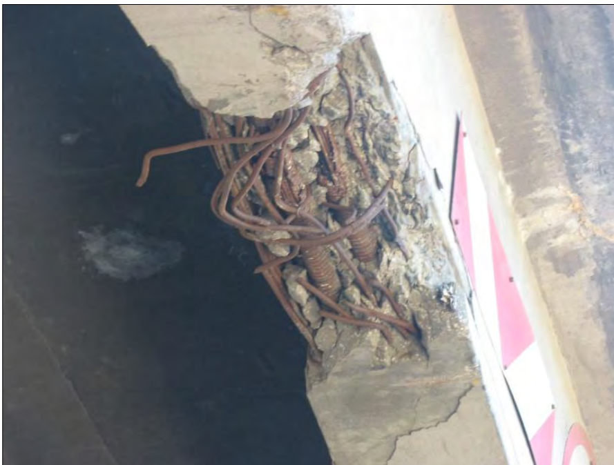
Figure 1: Bridge beam damaged as a result of transverse vehicular impact (SMEC, 2007)
