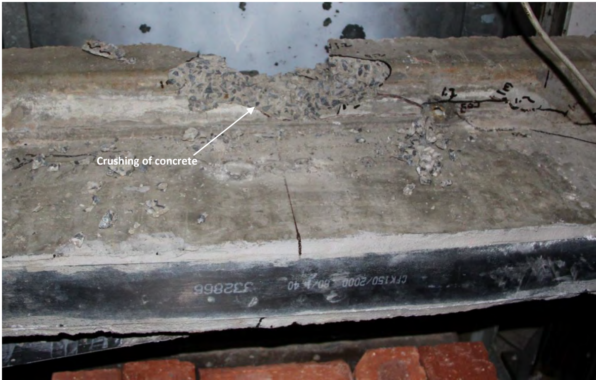
Figure B14: Compression damage and local damage (beam RS-80)
