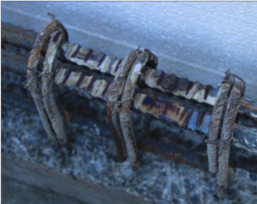
Figure 46: Reduced cross-sectional area of steel reinforcement
