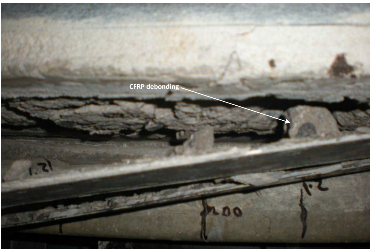
Figure B15: Debonding of additional CFRP applied for horizontal strengthening (beam RS-80)
