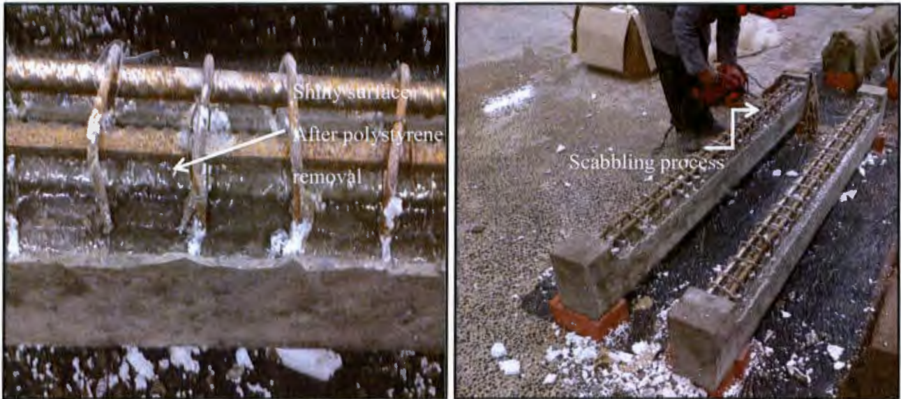
Figure 3.10 Concrete surface after the removal of polystyrene (left) and surface preparation by the scabbling process (right)
