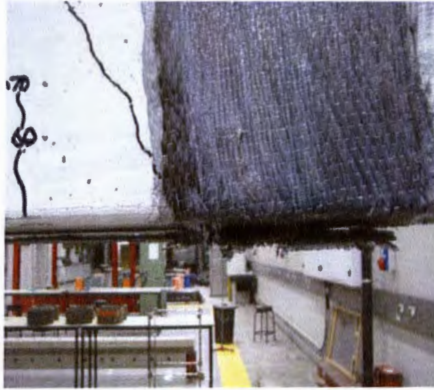
Figure D.1: Fractured FRP wrap near the right end support (beam S1.2)
