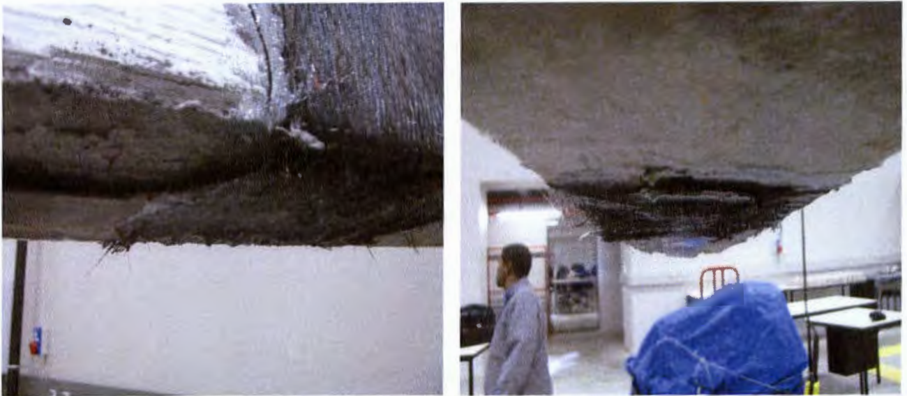
Figure D.2: Debonding of FRP wrap with partial fracturing of FRP wrap (BeamS3.4)
