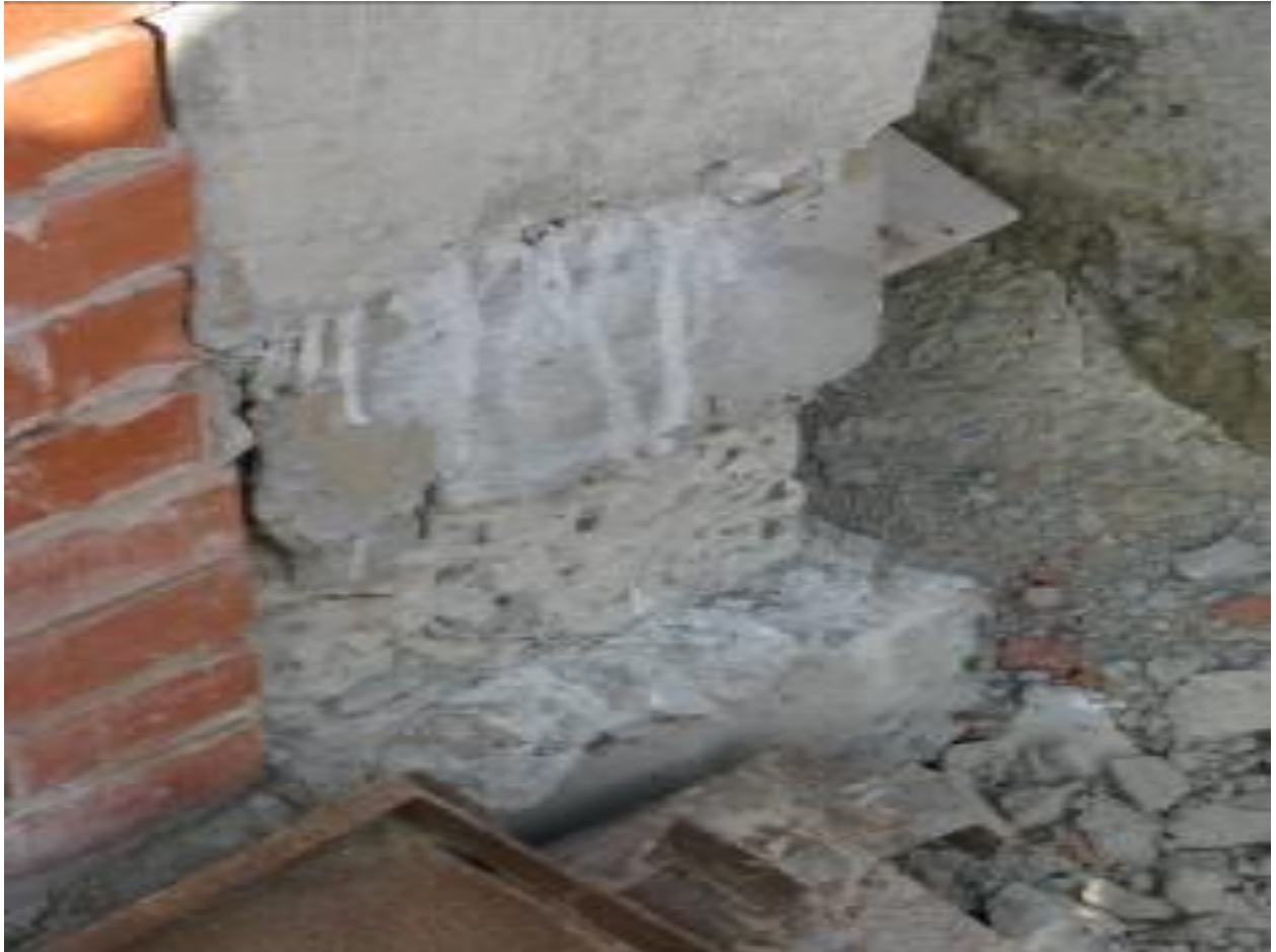
Appendix 1: Photograph depicts example of sub-standard work, e.g. support beams that have structurally been weakened, and poor brickwork.
