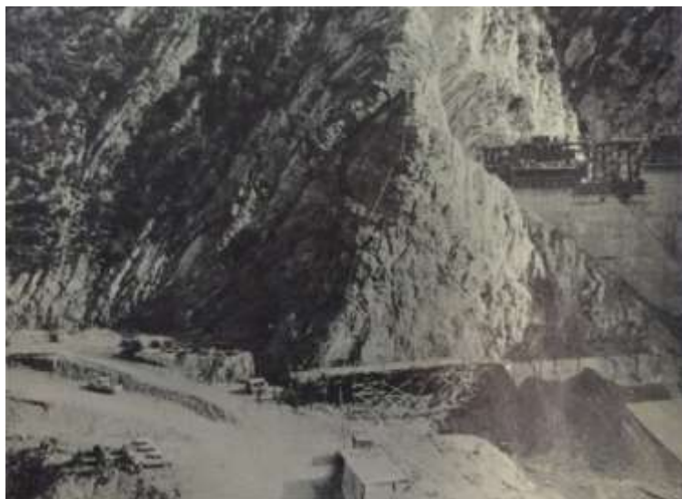
Figure 16: Right flank prior to completion and stress pad remedial measures (Hobbs et. al., 1967: 654)
