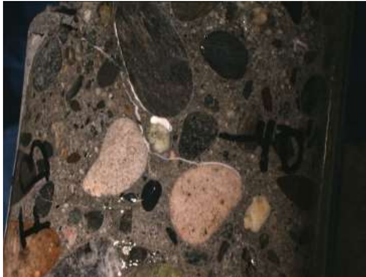
Figure 11: Cored sample of ASR deteriorated concrete (Concrete Microscope Library, 2016)
