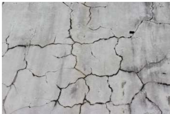
Figure 10: Classic ASR induced map cracking (Poraver, 2016)
