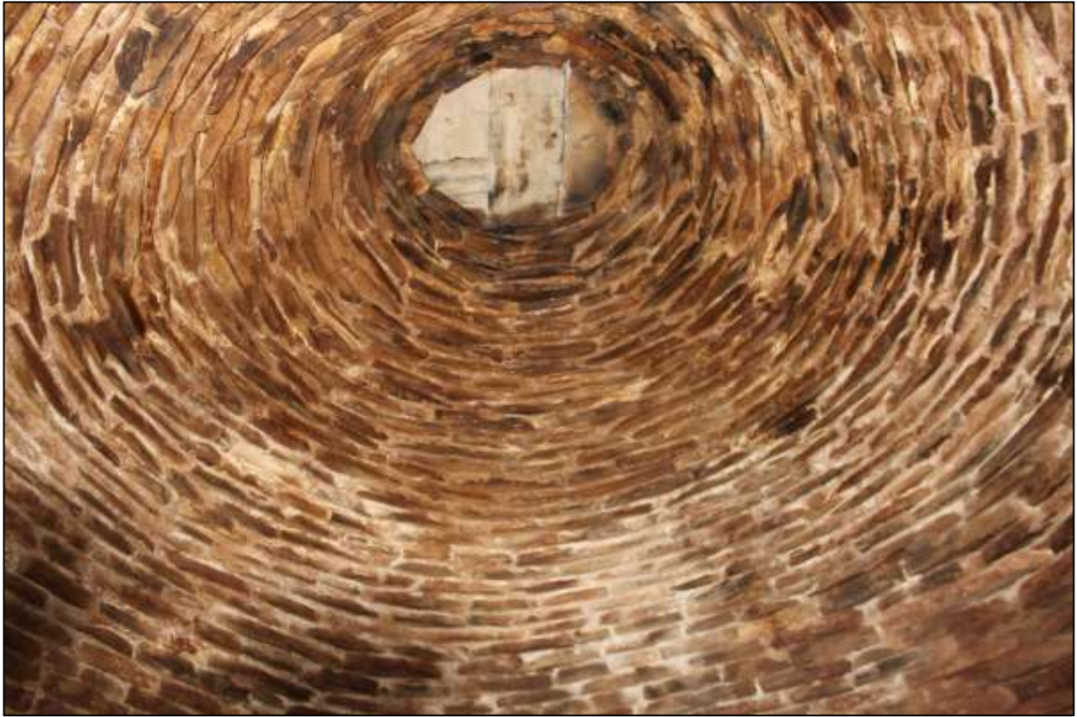
Figure 18 Photograph of the ceiling of a corbelled building on Osfontein farm showing the corbelling technique used in the Karoo.
