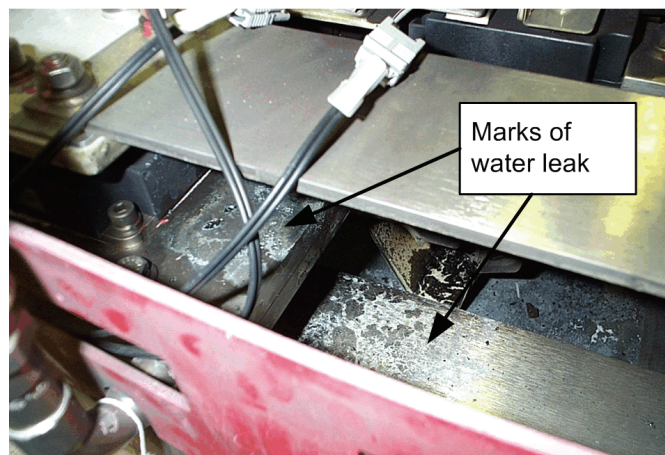
Fig. 6.20 Power Cell A2 showing water marks
