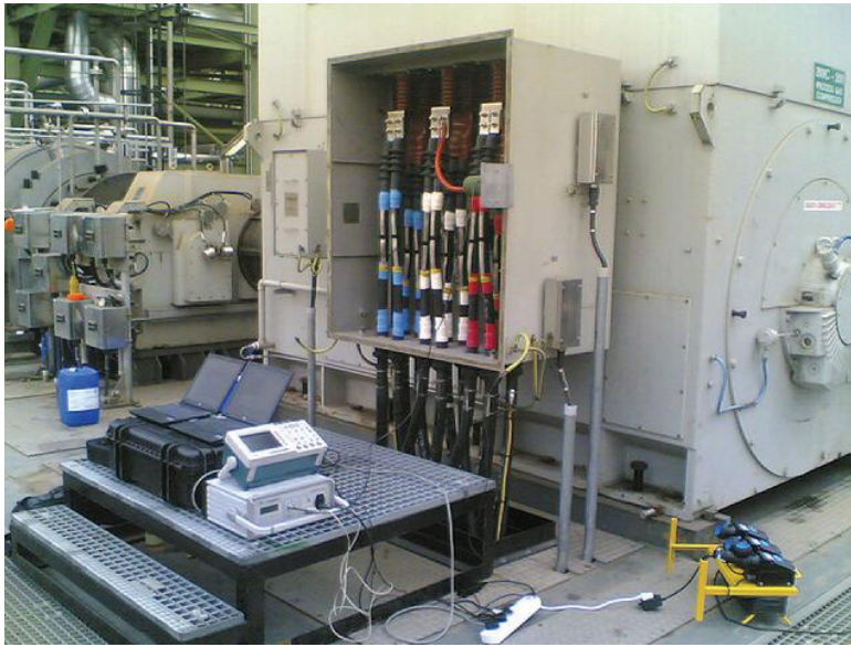
Fig. 2.8 Synchronous motor during site testing
