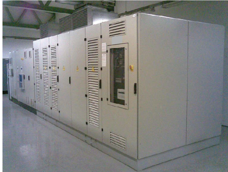
Fig. 2.14 12 pulse LCI (right), excitation and control panels (left)
