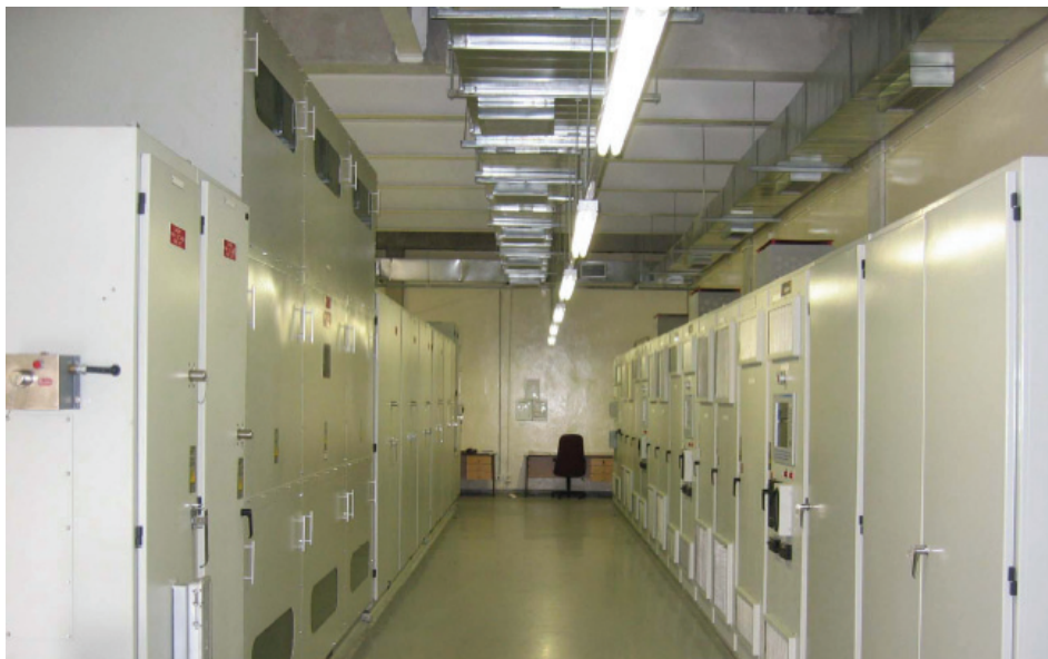
Fig. 2.7 Adjustable speed drive (left), excitation and control panels (right)
