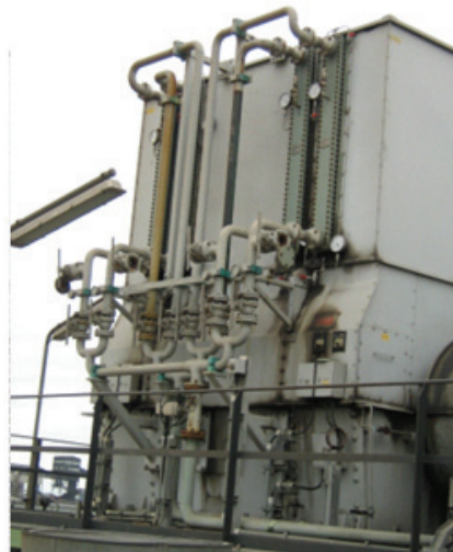
Fig. 2.15 Main Air Compressor (MAC) 55 MW Motor
