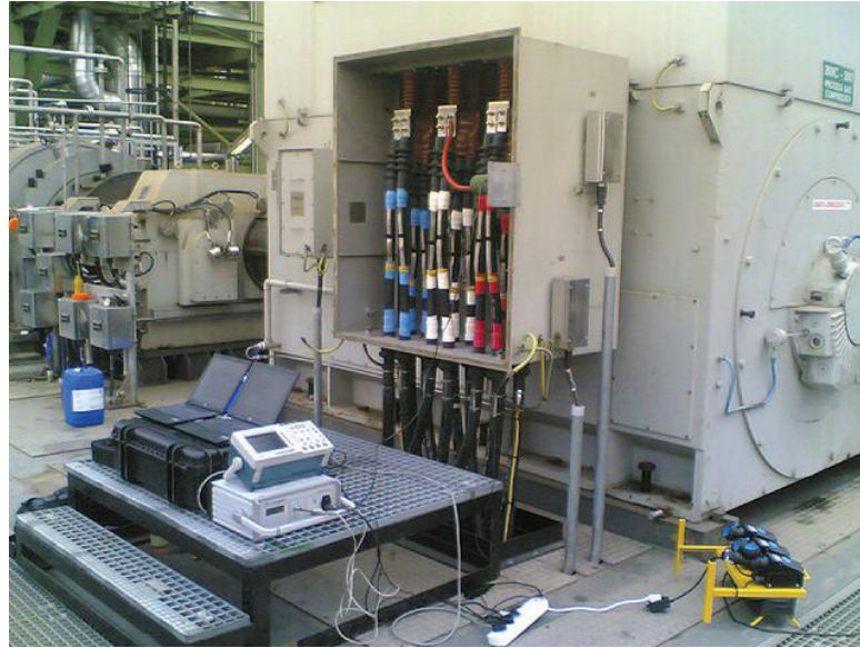
Fig. 3.8. Test set-up at the motor terminals
