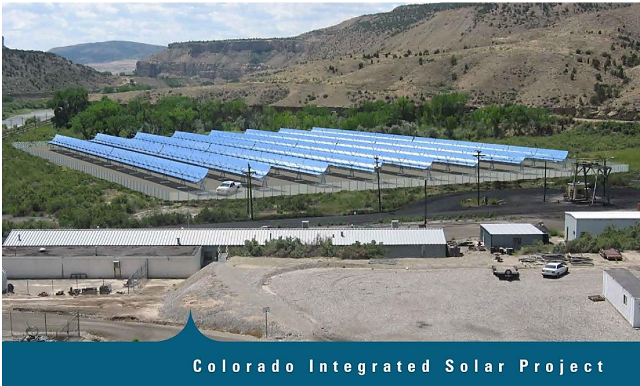
Figure 6: Cameo Generating Station SAPG system [15]
