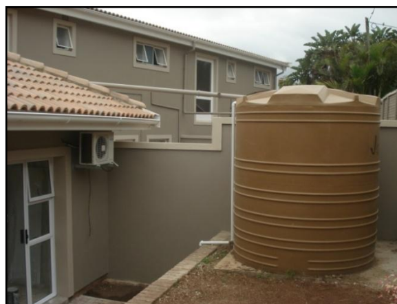
Figure 2.7: Rainwater harvesting tank, Selborne Estate, East London
