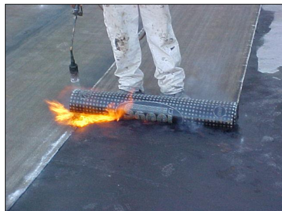
Figure 3.2: Waterproofing a roof in preparation for the construction of a green roof
