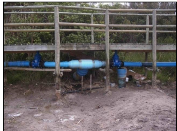
Figure 5.10: Treated effluent inlet into Cell 1
