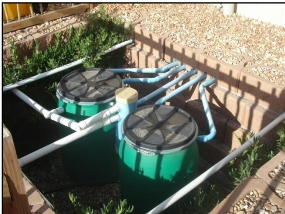
Figure 4.34: Greywater digesters used daily at eco-centre
