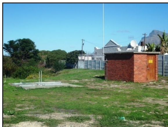
Figure 4.24: Wingfield outfall pump station and hydraulic testing pit
