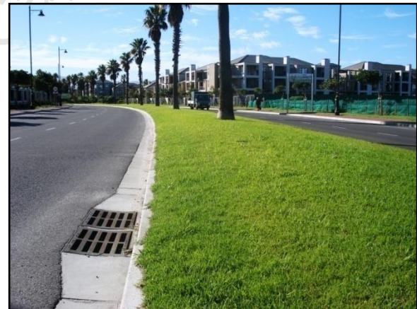
Figure 5.8: Conventional cast iron catchpit situated at foot of filter strip
