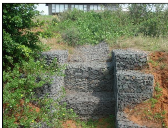
Figure 2.16: Gabion structure utilised as erosion protection inlet, eThekweni
