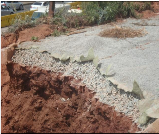
Figure 4.6: Section through the base layers that will support permeable concrete block pavers
