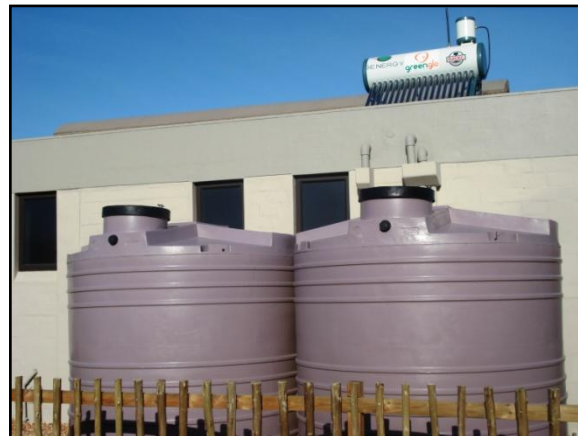
Figure 4.8: Solar powered stormwater collection and reuse system
