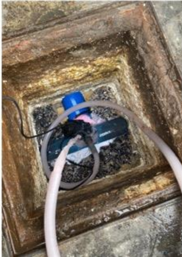
Figure 3.3 | Pumping of raw DWW
