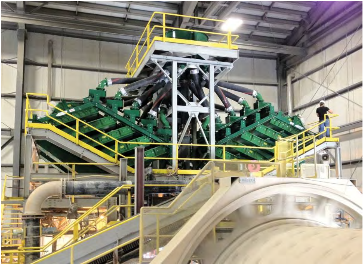
Figure 2-3 Derrick stack sizer unit in operation (courtesy: Derrick corporation)
