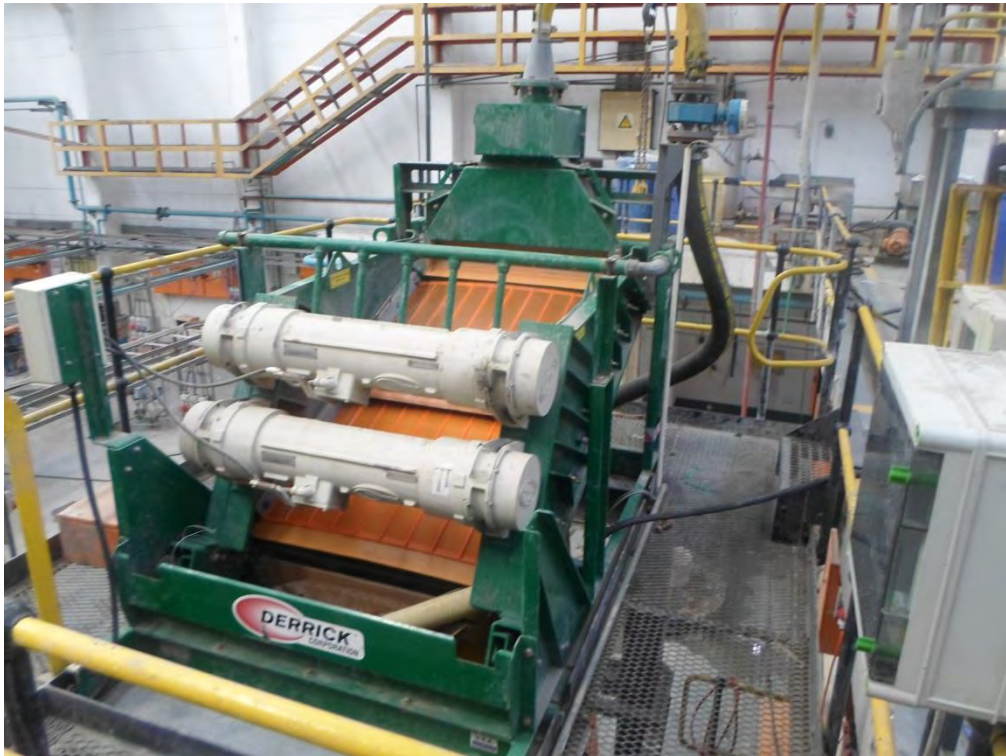
Figure 3-1 Single deck Derrick screen installed at Mintek
