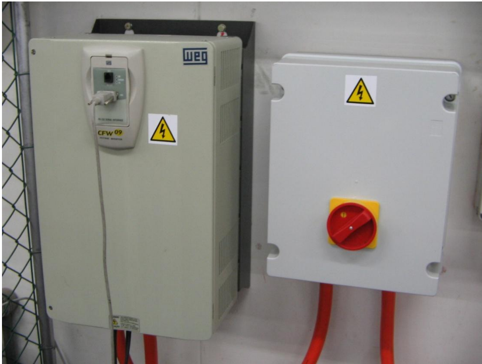
Figure 96: VSD Mounted on Wall
