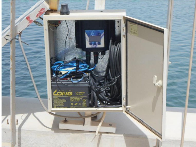
Figure 26 is the inside of the electronics box, Abu Dhabi as described below (2015).
