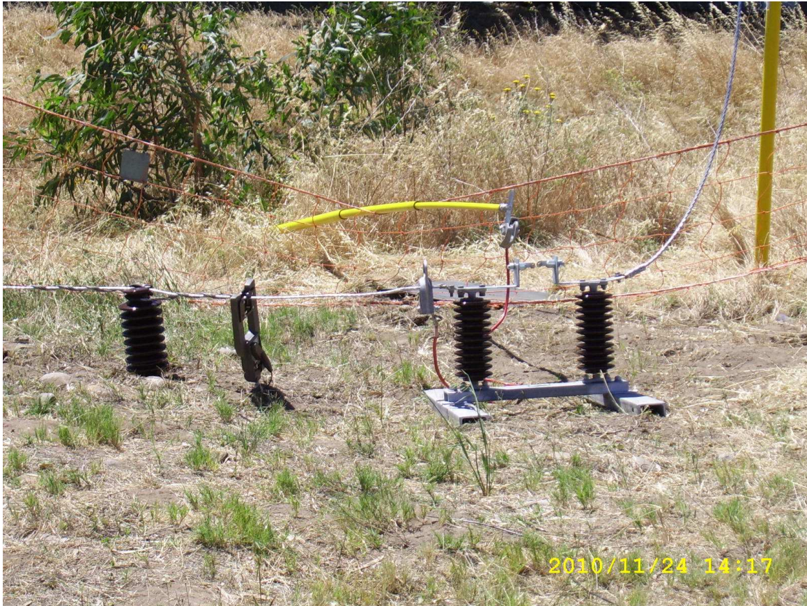
Figure 28: The actual arcing horn purposely built to facilitate the fault throws in order to verify operation of the TEFCS.
