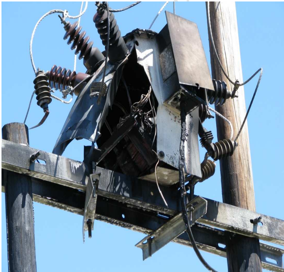
Figure 26: Failed CT/VT metering unit.
