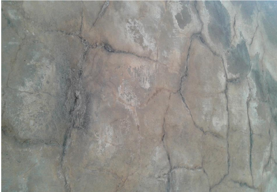
Figure 1 ASR wider and spreading map pattern cracks (Wood, 2009)
