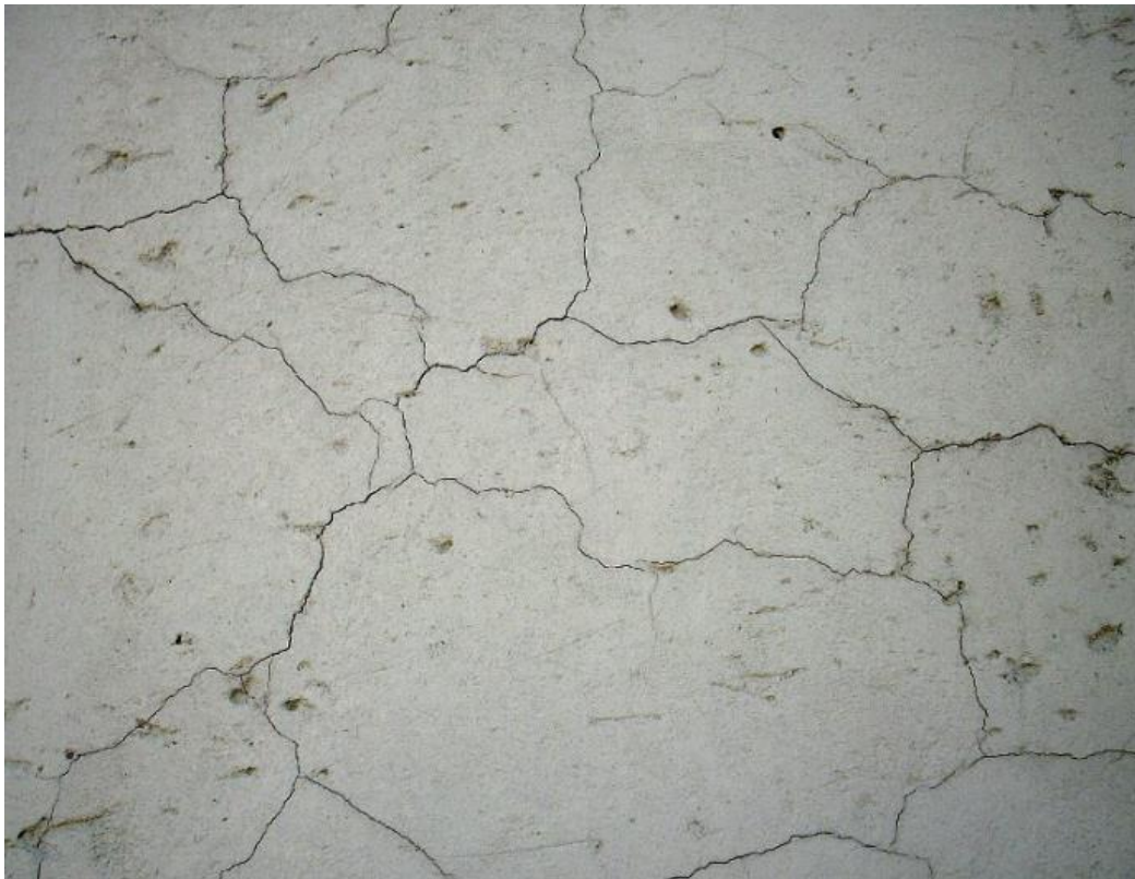
Figure 7: Map pattern cracks (CRM1-279, 2012)
