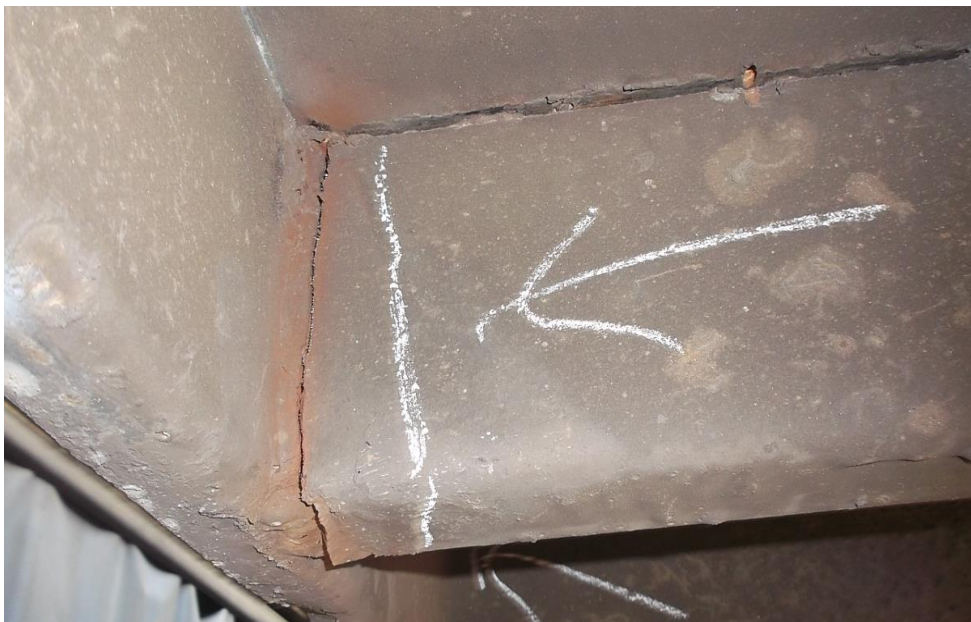
Figure 5: Structural cracks (Edwin, 2017)
