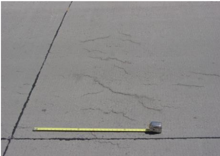
Figure 3: Plastic shrinkage cracks at Unilever Ice Cream Plant in Midrand, Johannesburg
