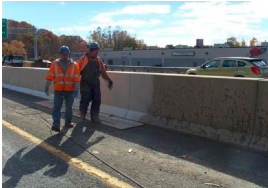
Figure 27: Typical ASR damage on barrier walls treated with elastomeric coating at Massachusetts site (Michael et.al, 2013)
