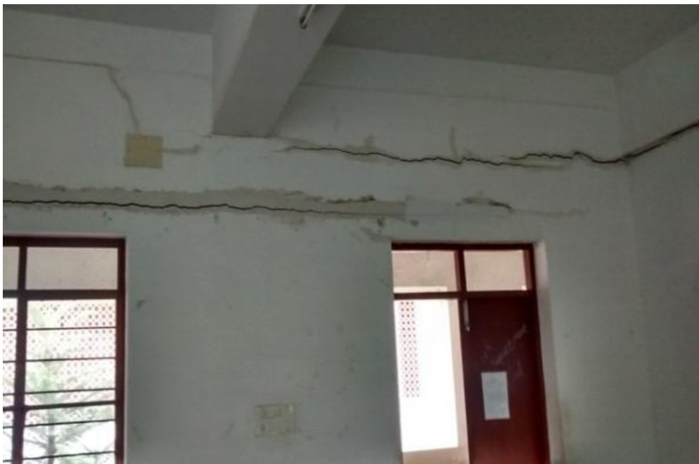
Figure 6: Structural cracks at Phephetso Secondary School classrooms
