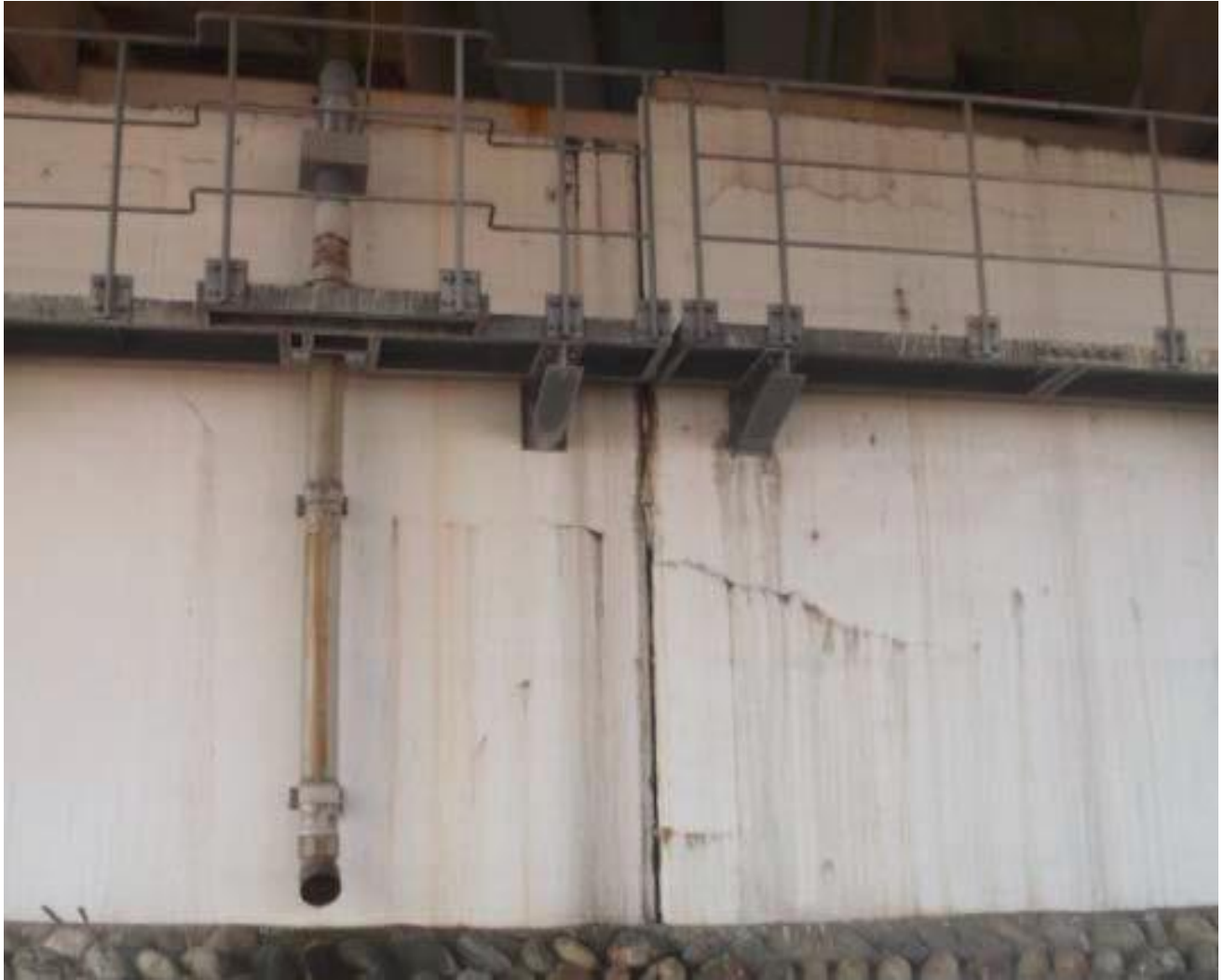
Figure 29: Cracks occurred on the repaired structure (Nomura et.al, 2012)
