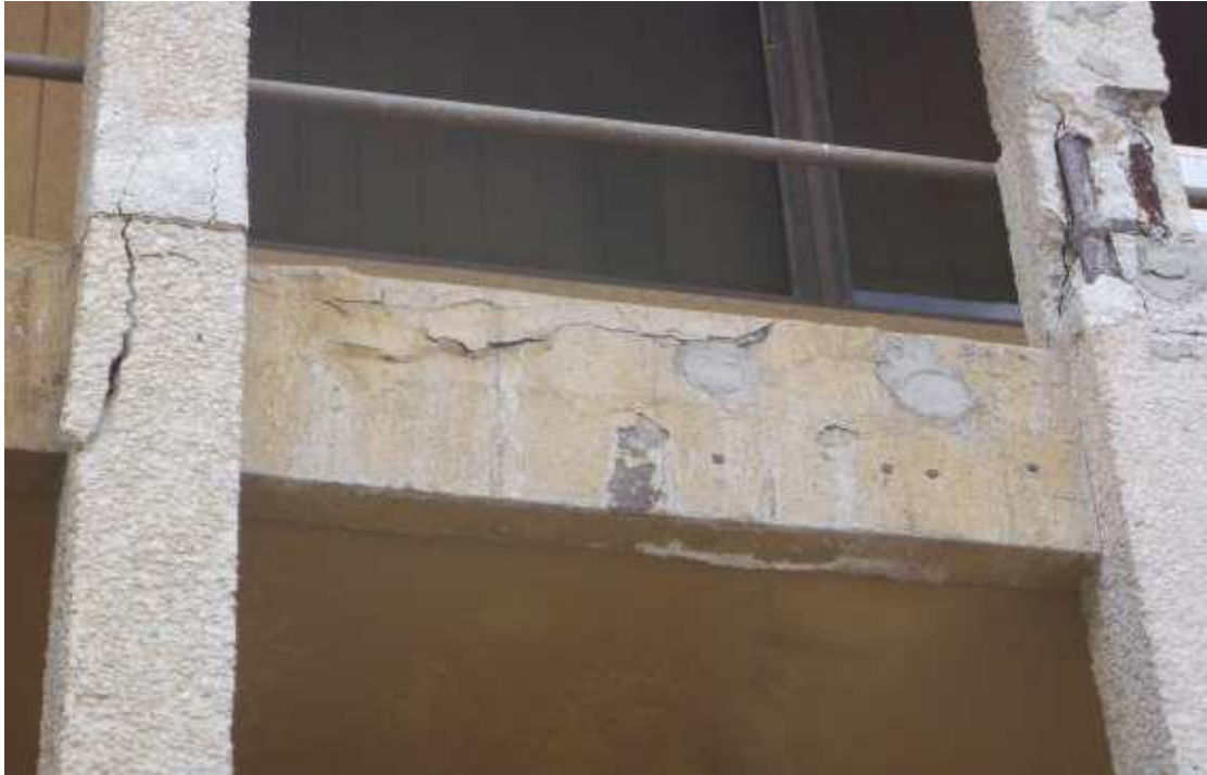
Figure 2: Cracking, spalling and delaminations at the SABS building due to corrosion effects
