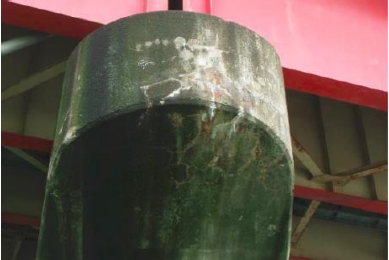
Figure 28: Deterioration due to ASR (Nomura, M., et.al, 2012)
