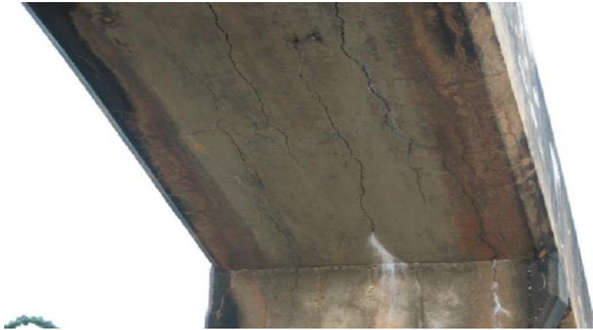
Figure 25: Cracking on top and underside of archway supporting the 5th span (Michael et.al, 2013)
