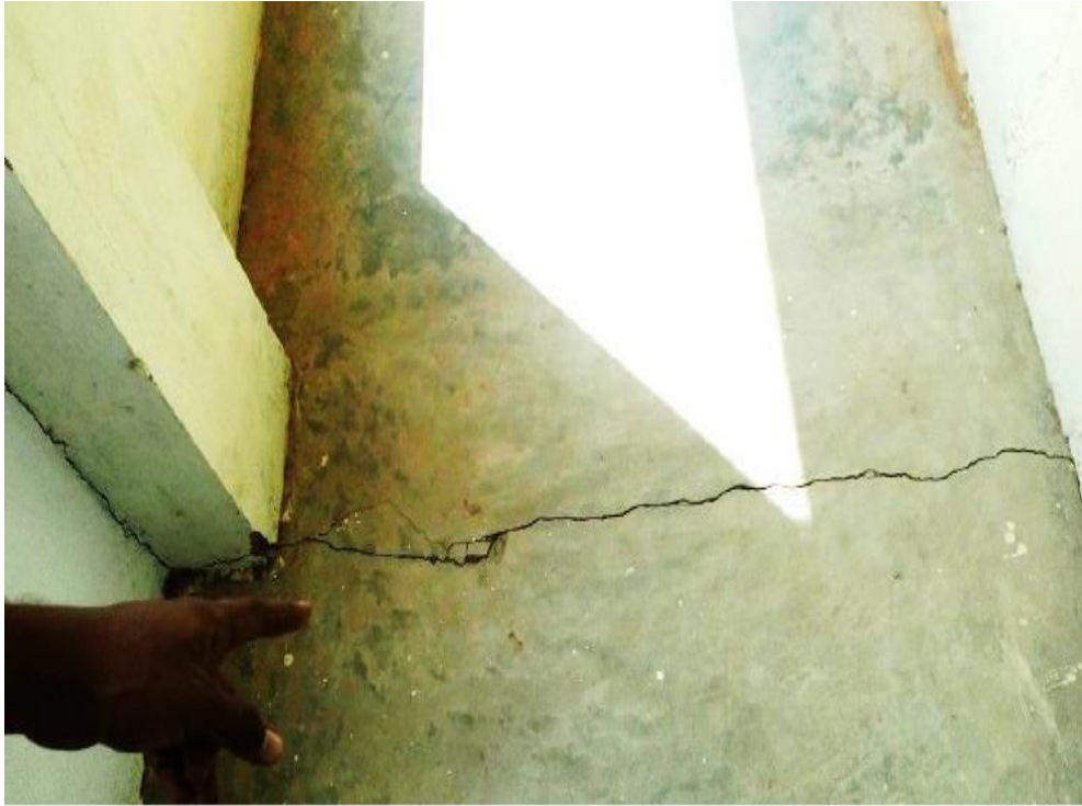
Figure 32: Drying shrinkage cracks within the parking structure (Sika, 2016)
