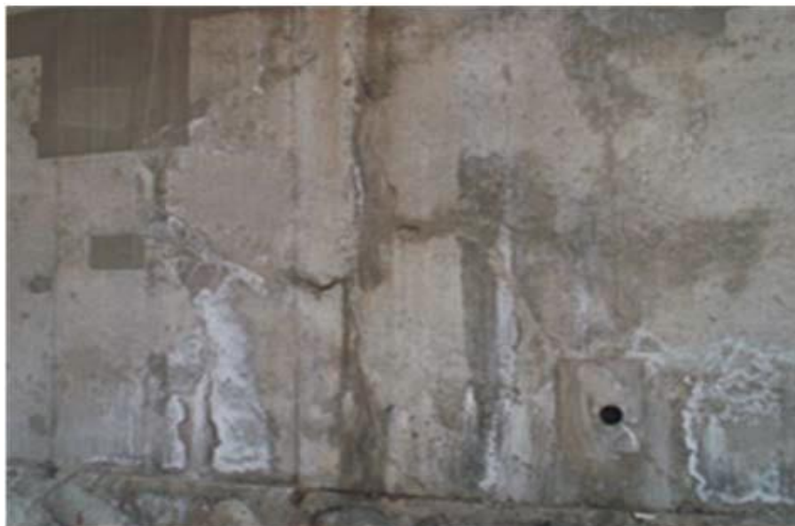
Figure 31: Cracks occurred on the patch repair structure H (Nomura, et.al, 2012)
