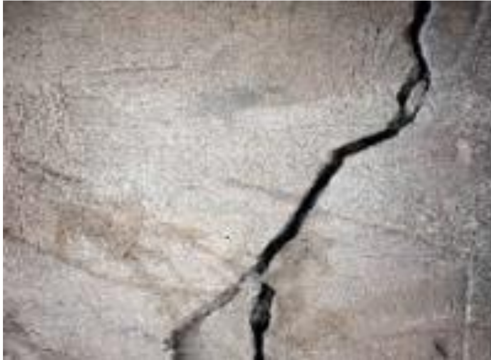
Figure 9: Offset cracking (CRM1-279, 2012)
