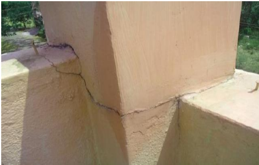
Figure 35: Structural cracks starting to appear due to accidental loading (Trout, 2006)
