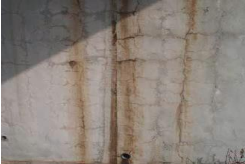
Figure 30: Cracks occurred on the patch repair in structure F (Nomura, et.al, 2012)
