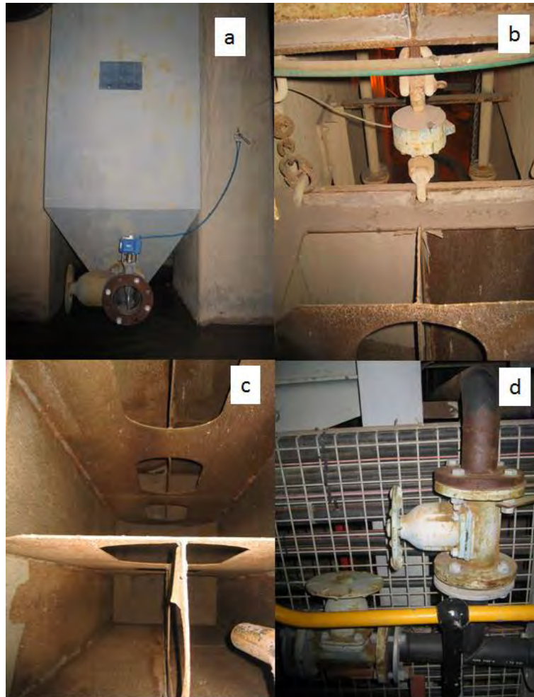
Figure 19: Concentrate drop tank on Stream s8 showing (a) the drain valve, (b) mechanical support, (c) top view and (d) by-pass valve
