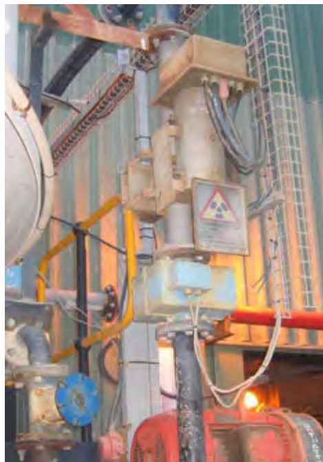
Figure 18: Magnetic flow meter and densitometer assembly on Stream s8
