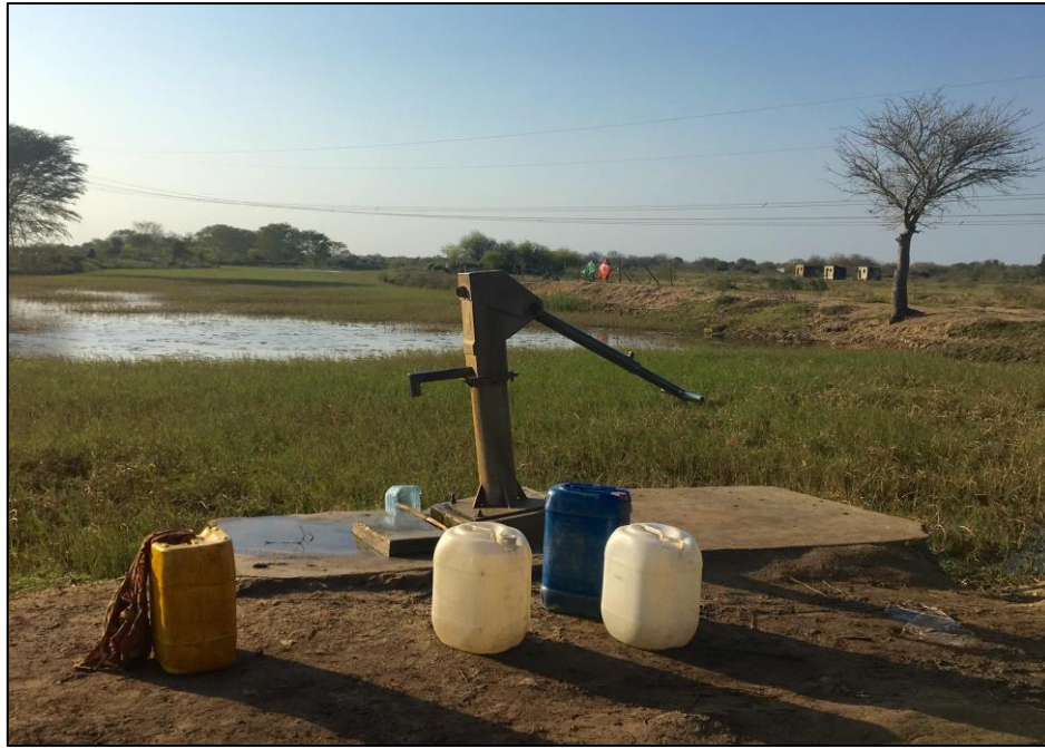
Figure 2-1 Example of a community hand pump in Southern Mozambique.
