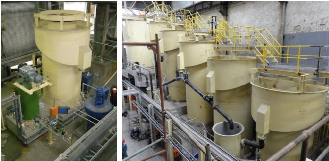
Figure 2.5: Staged Flotation Reactor (Courtesy Woodgrove Technologies Inc., 2015)
