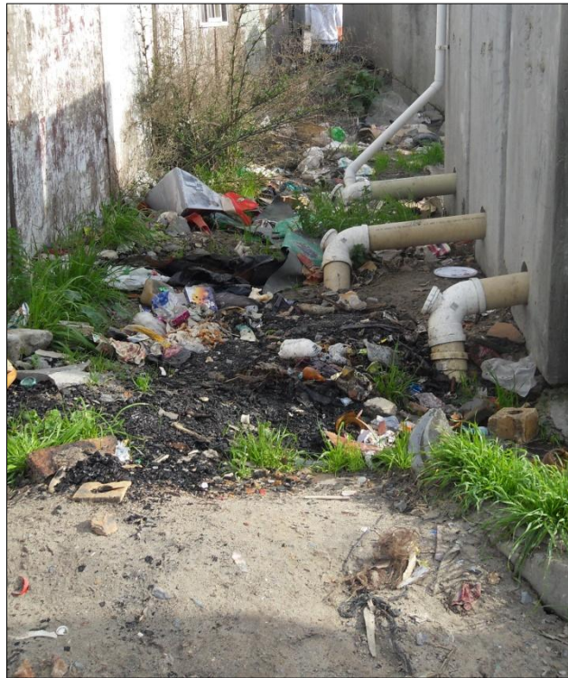
Figure 6: Rubbish strewn behind public toilets, Cloverdale
