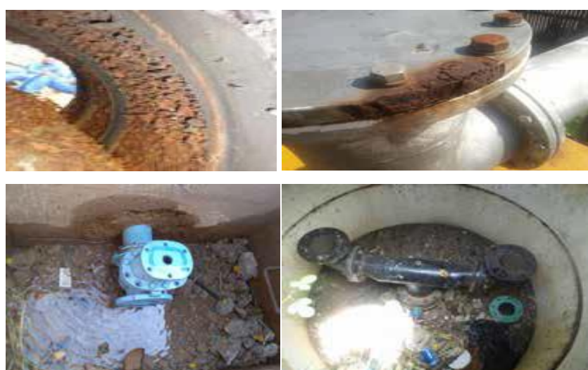
Figure 2.14: Examples of pipe loss of physical integrity (Adapted from Armitage, 2015)
