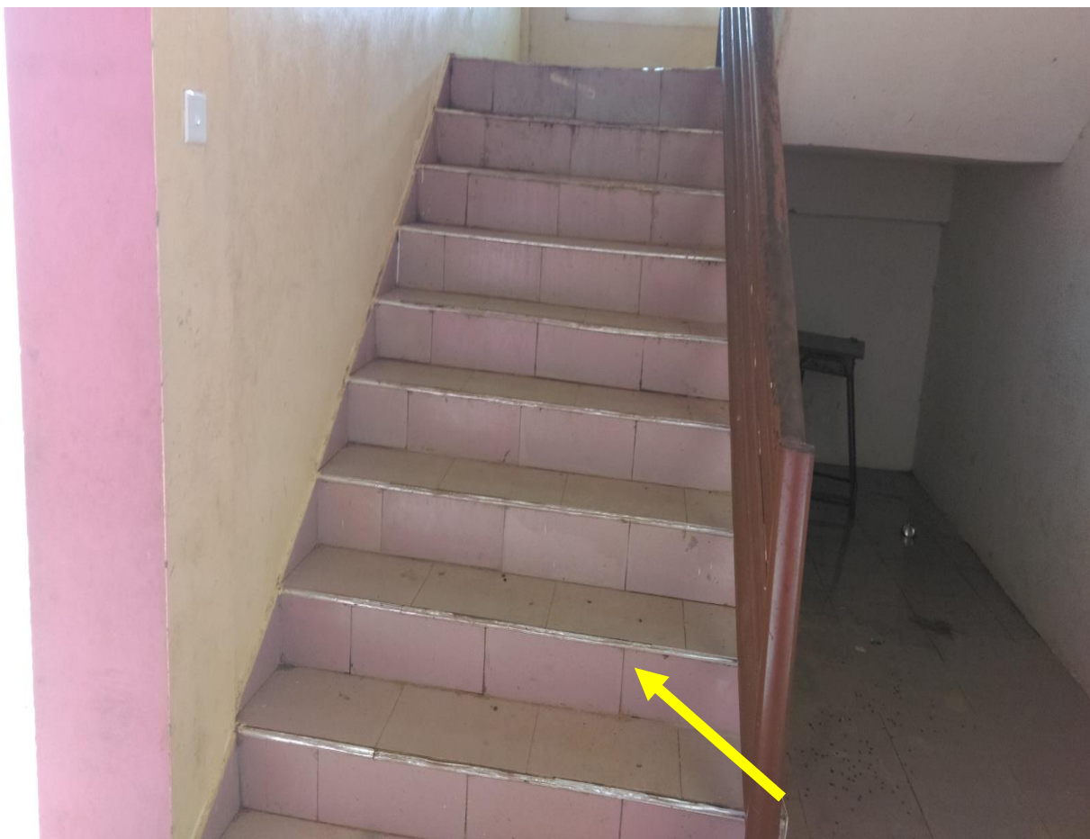
Figure 6 A staircase leading to the classrooms on the top floor in the KSC
