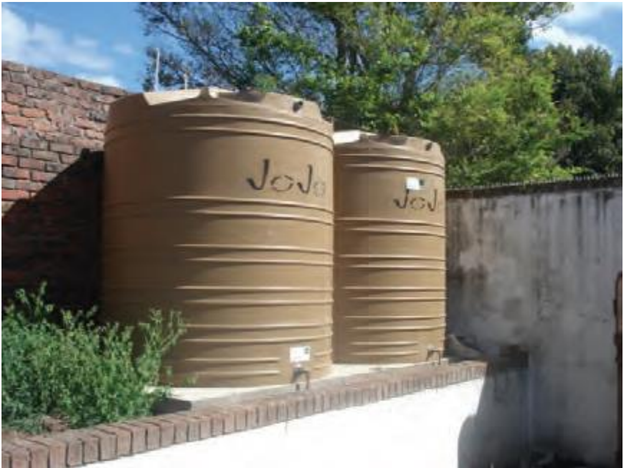
Figure 33, Roof runoff storage tanks (Armitage et al, 2013)
