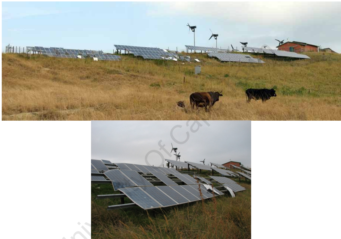
Figure B-7: The Lucingweni hybrid mini-grid system in May 2007, shortly after it was vandalised. Around 40% of the total PV panels were either stolen or inoperable due to vandalism.
