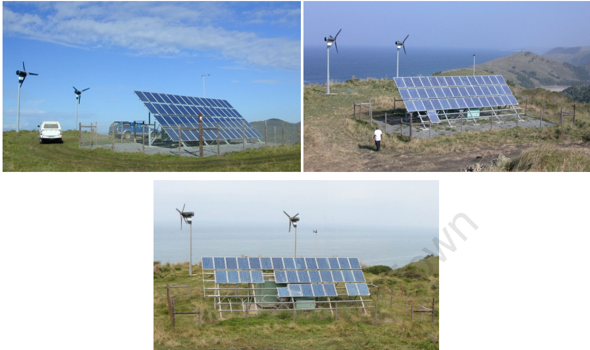
Figure 2-6: The PV array at Hluleka, photographed in June 2003 (top left), July 2006 (top right) and May 2007 (bottom). July 2006 photograph by C. T. Gaunt (reproduced from Appendix B)
