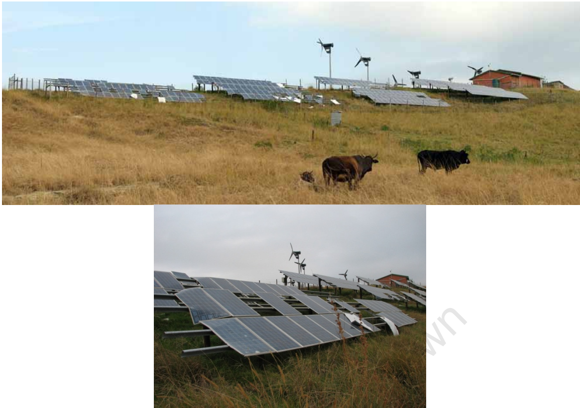
Figure 1-4: The Lucingweni hybrid mini-grid system in May 2007. Around 40% of the total PV panels were either stolen or inoperable due to vandalism.
