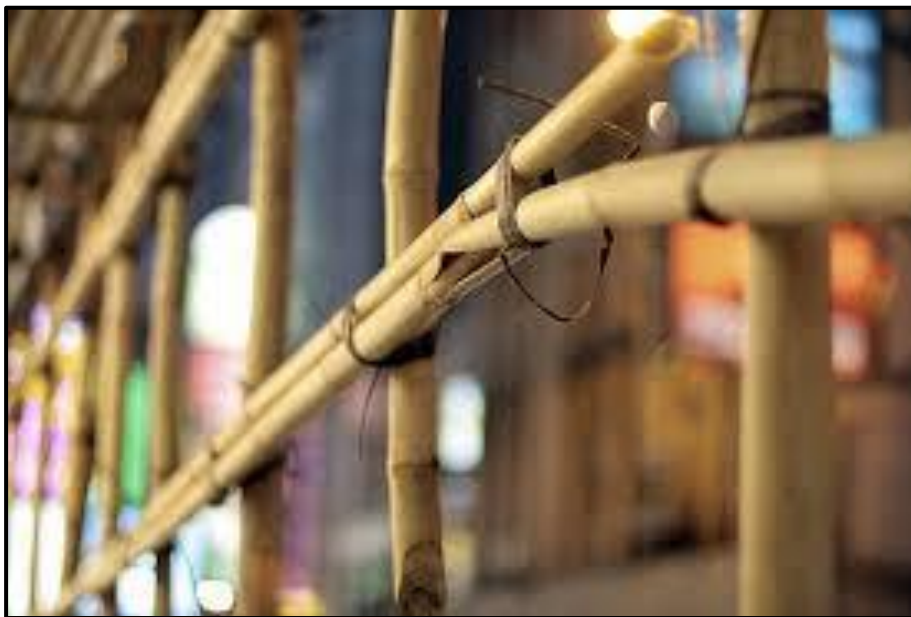
Figure 4.4: Typical splitting failure in bamboo culms (Janssen, 2000)
