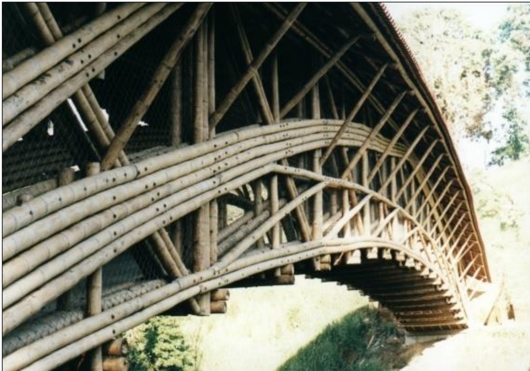
Figure 6.19: Insufficient arching of the bridge (Stamm, 2004)
