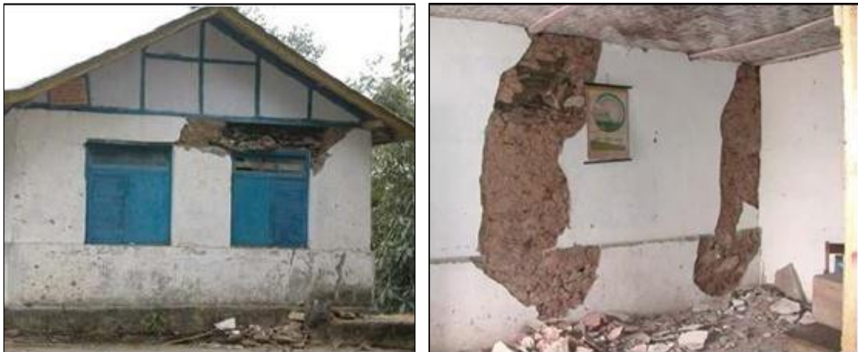
Figure 5.30: Damaged masonry building following the Sikkim earthquake, India (Sharma, 2010)
