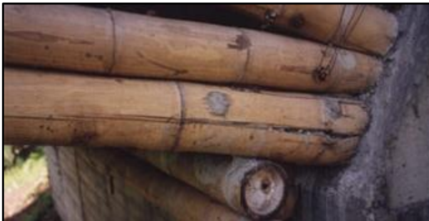
Figure 4.7: Failure in shear in the direction of fibres (Tönges, 2002)
