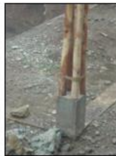
(d) Reinforced concrete column plinths with four bamboo culms forming one column
