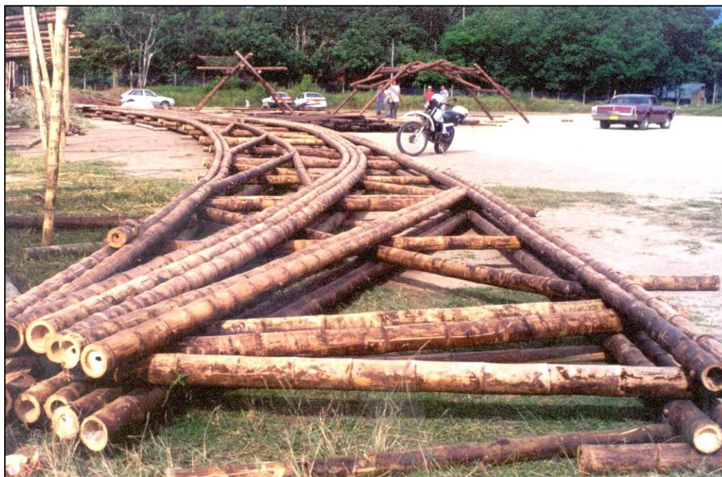
Figure 6.13: Typical construction of bamboo trusses for the Liceo Frances Arch Bridge (Stamm, 2004)
