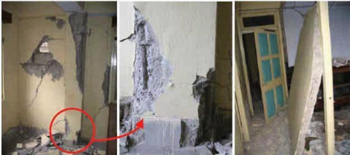
Figure 5.31: Damage to a reinforced concrete building following the Sikkim earthquake (Sharma, 2010)
