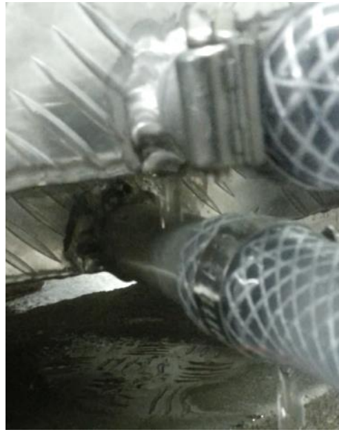
Figure 4-27: Leakage at drainage outlets
