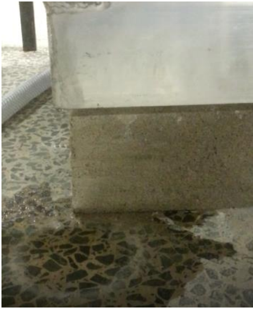
Figure 4-26 Minor Leak at the bottom of tank
