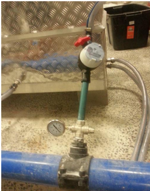
Figure 3-7 : Delivery pipe connected to PRV and Flow meter
