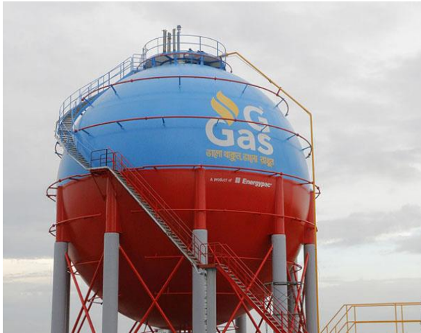
Figure 1-1: spherical vessel with liquefied gas [https://www.marksanglobal.com/oil-gas-storage.php]
