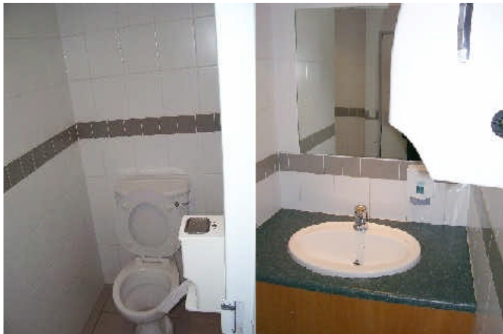
Figure 23 Private Hospital Ablutions
